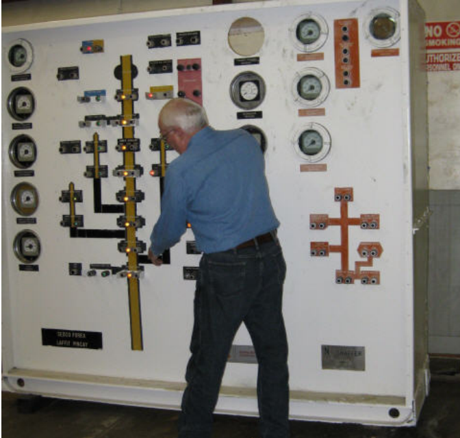
Control panel for subsea control unit
