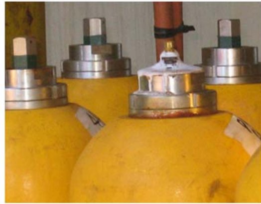
Figure 2. Leaking Charge Valve.
